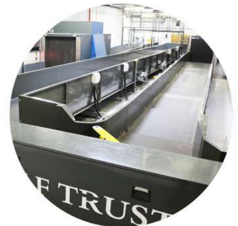
Baggage Handling Systems
